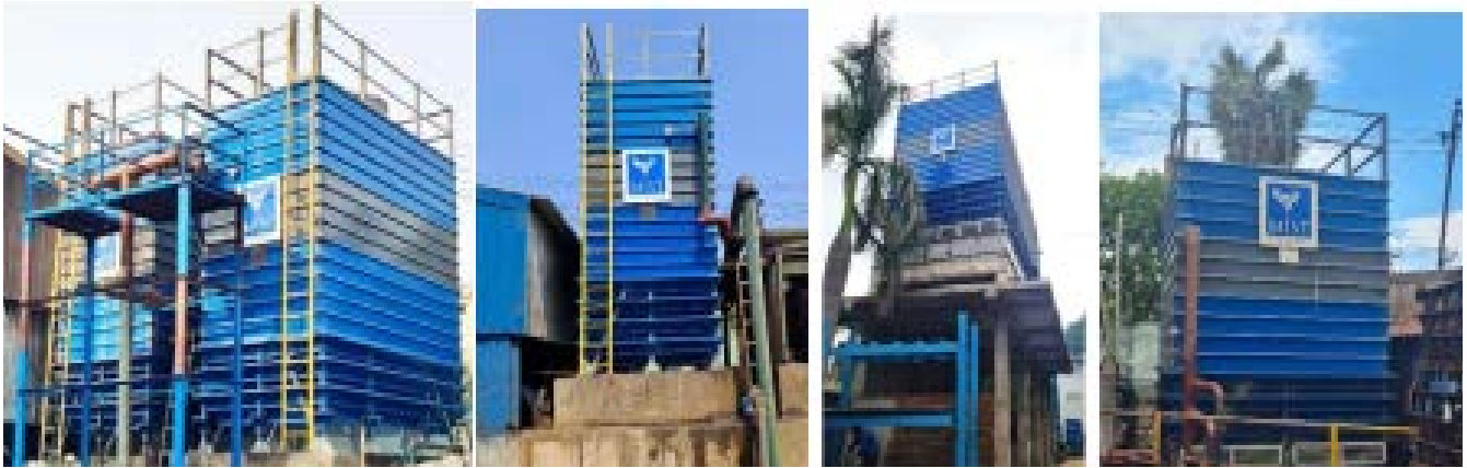
Figure 35 New induced draft mist cooling towers at M/s.RKFL
