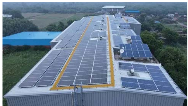
Figure 26 Solar Panels on Roof Top
