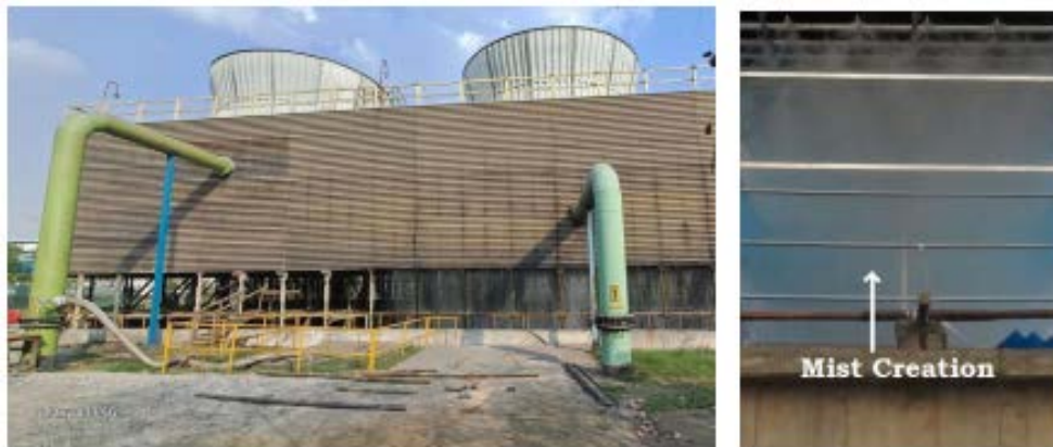
Figure 37 New IDMCT pictures at M/S. Vedanta Ltd. after refurbishment
