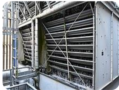
Figure 7: Cooling Tower in Plant
