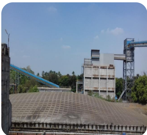
Figure 6: Lagoon in place at SPB, Erode
