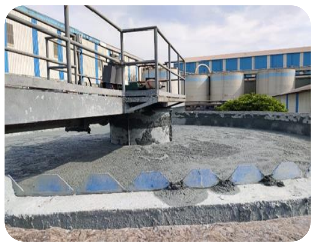
Figure 11: 9m clarifier unit
