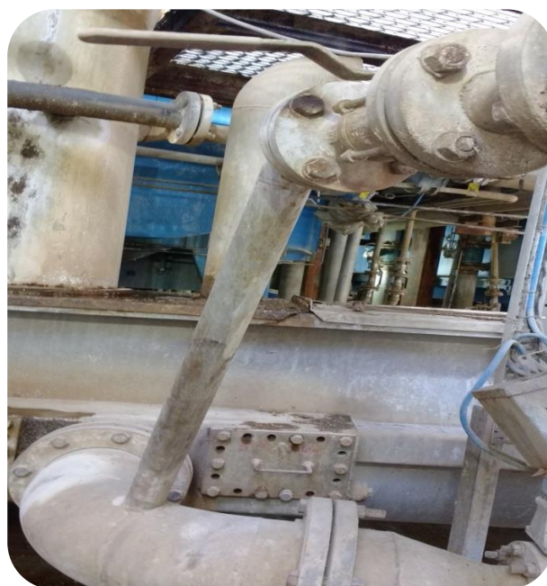
Figure 1: NaOH Valve in closed condition
