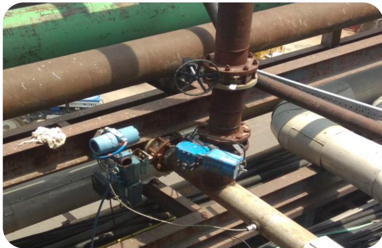
Figure 8: Arrangement made for recycling hot water
