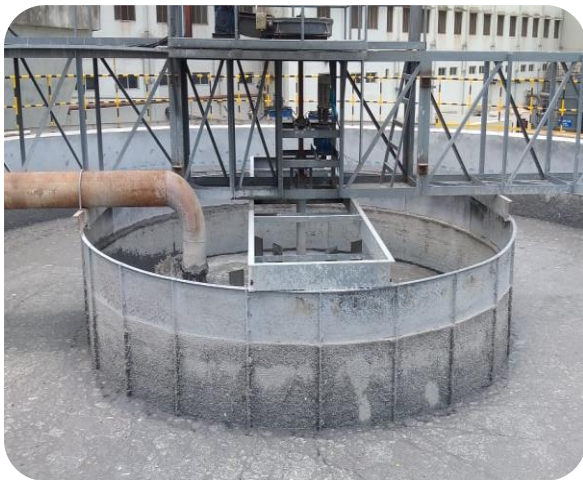
Figure 11: 20m clariflocculator unit
