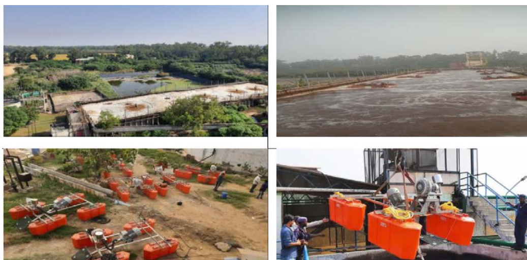
Figure 35 Old Surface Aerators and Turbo Oxy Jet Aerators cum Mixers 30+3 hp in aeration basin
