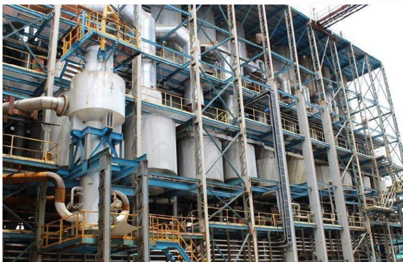
Figure 16 Chemical Recovery Plant
