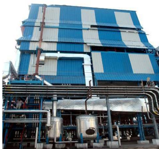
Figure 12 Boiler 10 AFBC -Coal fired HP Boiler
