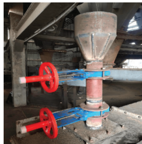
Figure 10 Feeding system for Oxy-booster
