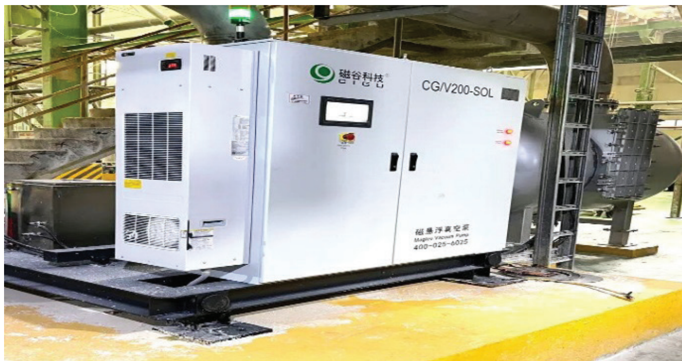
Figure 7 Installed CIGU maglev turbine vacuum pumps at APP Indonesia
