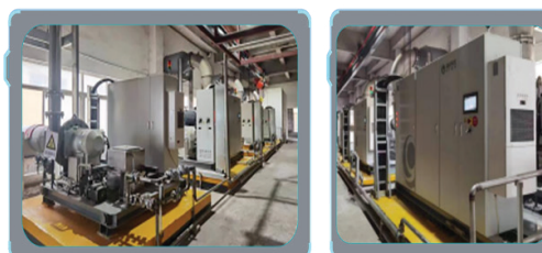
Figure 4 Installed CIGU maglev turbine vacuum pumps at the Yueyang mill, with the before/after cost comparison
